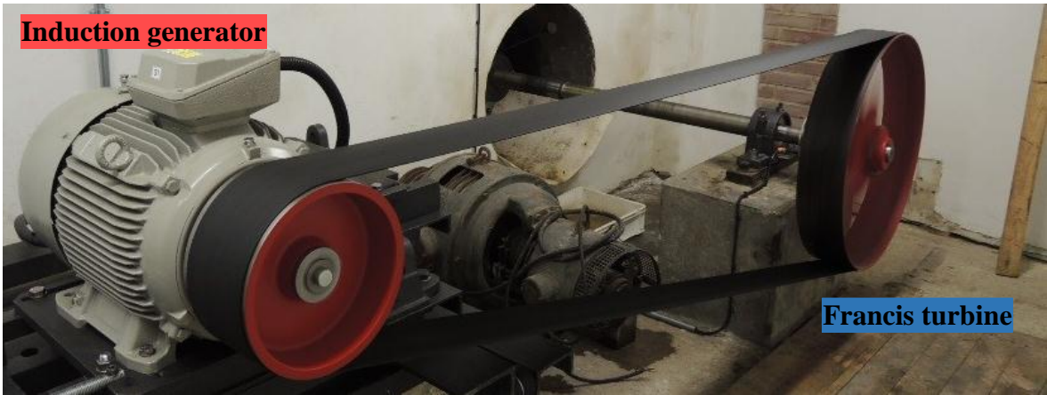
Figure 1 View on the generator and output shaft of the small hydro power plant
