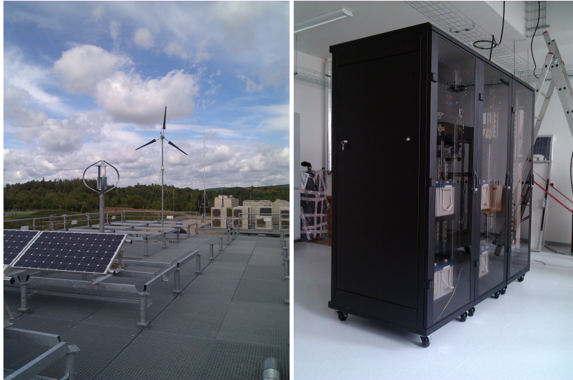
Figure 1: Experimental hybrid energy system and the control room
